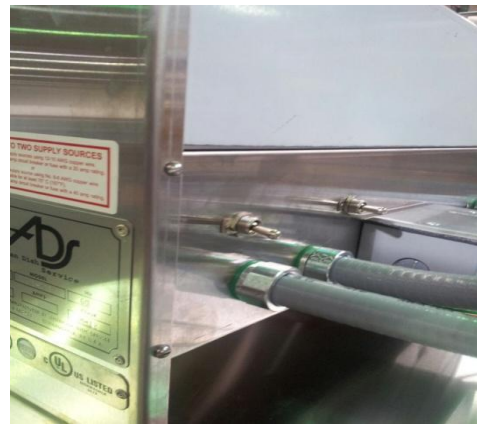
Showing the two master switches
