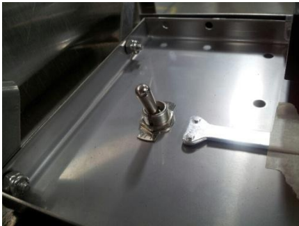
De-lime switch in control box
