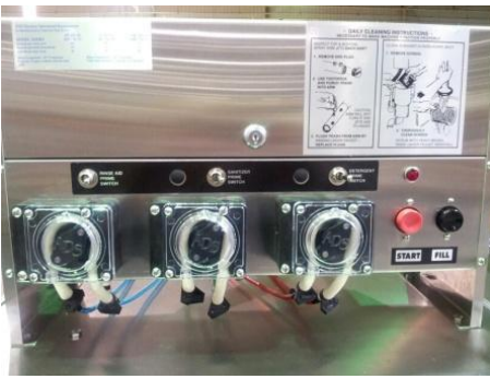
Showing deter, rinse, sanitizer external pumps
