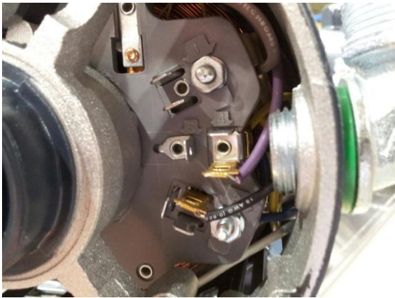
Showing connection points in 1.5 HP, 120v motor black & white wires attach to spades left of the two nuts
