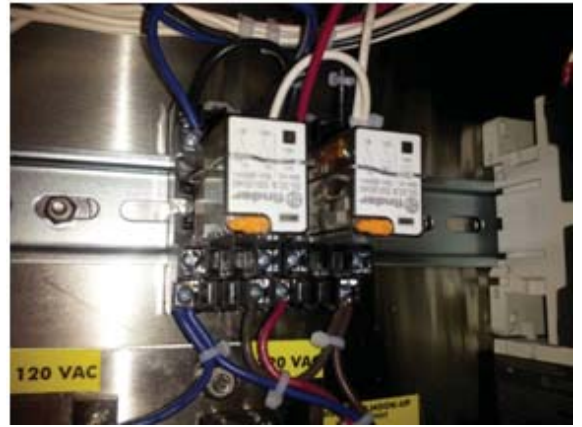
Conveyor motor control relays
