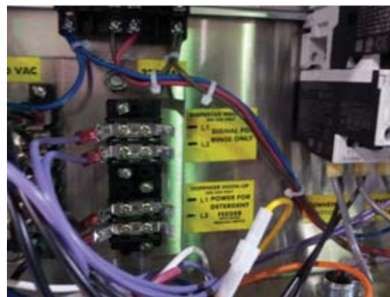
Dispenser signal connection terminals in control box
