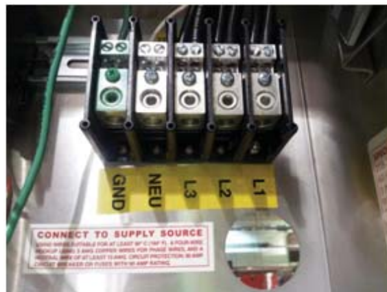
Main distribution block for 66's incoming 3-ph, note Neutral
