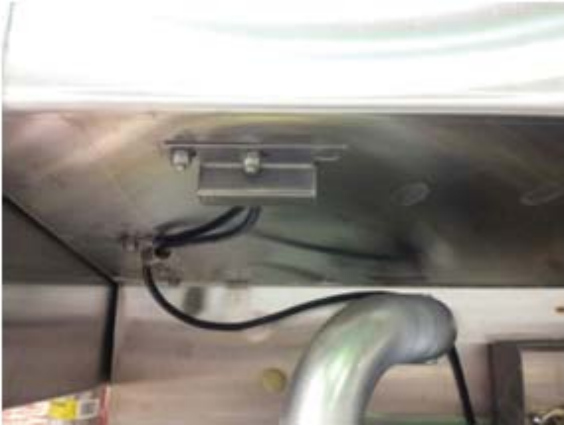
Sequence reed switch for wash tank
