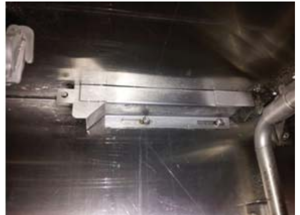
Showing “float” switch that controls fill water & heater
