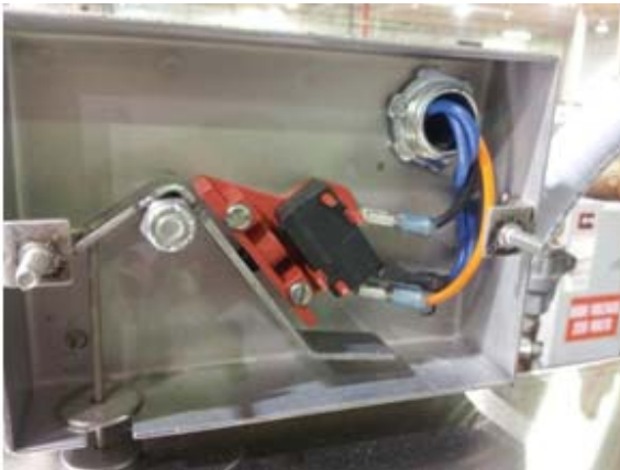
Showing “float” switch that controls fill water & heater
