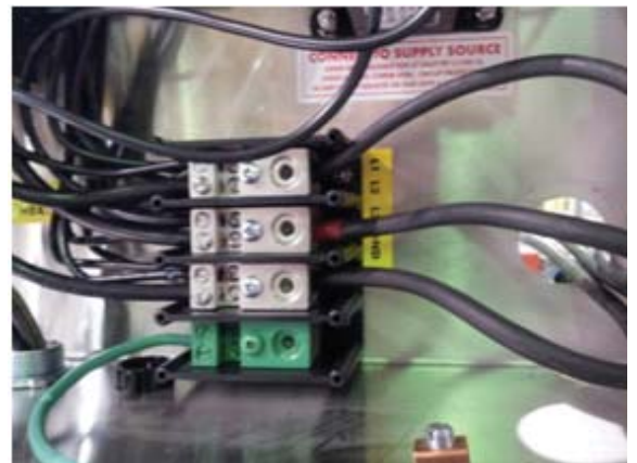
Main distribution block for 44's incoming 3-phase
