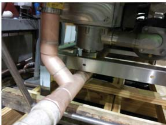
Showing 2" drain manifold exiting sump & scrap box
