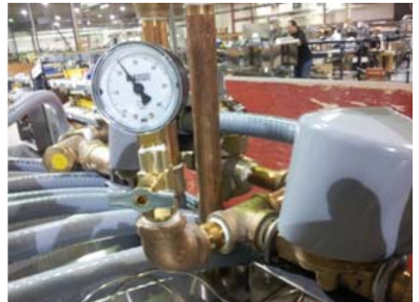
Final rinse manifold with pressure gauge, 20 psi flow req.
