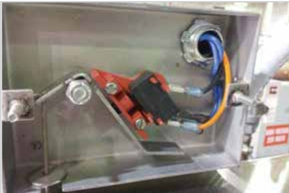
Showing "float" switch that controls fill water & heater
