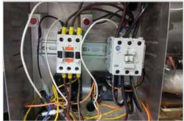
T-stat signal goes to term #6 on heater relay under contactor
