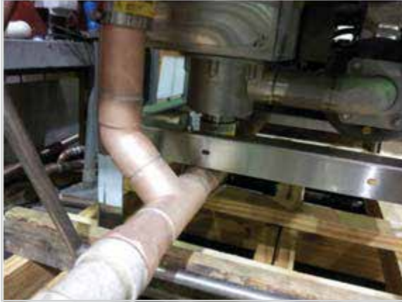
Showing 2" drain manifold exiting sump & scrap box
