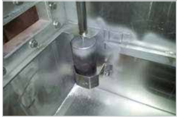
Wash tank float and tank overflow
