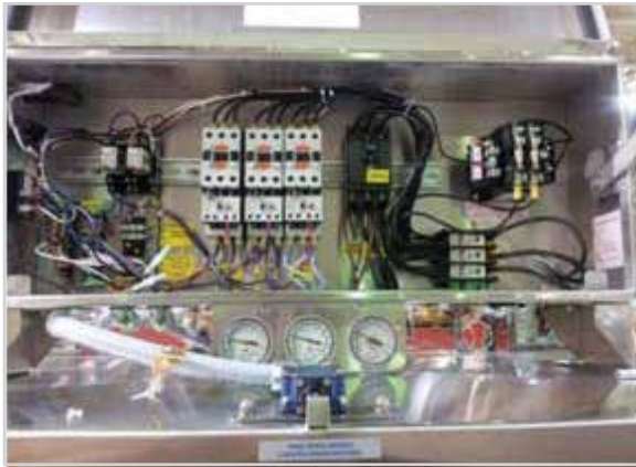
ADC-44 conveyor control box for 3-phase power
