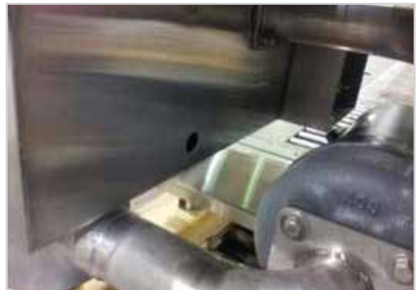
Showing 7/8" detergent probe hole behind pump motor
