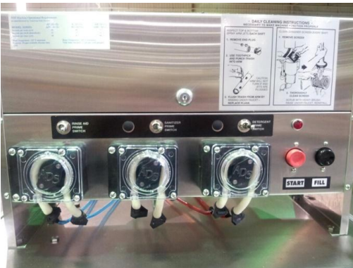
Showing chemical detergent, rinse, sanitizer external pumps
