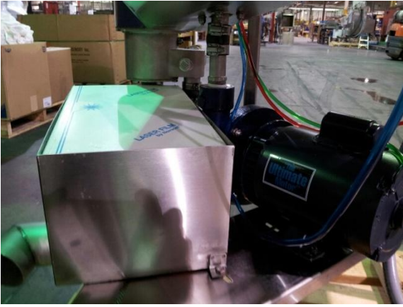
Rear view of installed side exit ES scrap box
