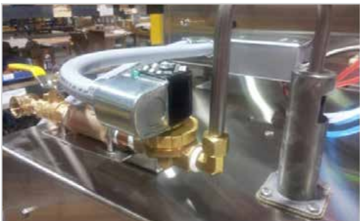
Showing 1/2" female pipe inlet, ball valve, y-line filter, water solenoid, ASSE approved air gap (backflow preventer)
