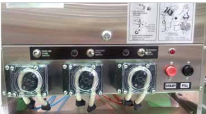
Showing chemical detergent, rinse, sanitizer external pumps
