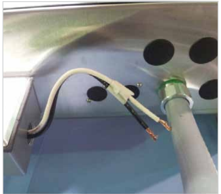
Showing power connection box for 120v wiring
