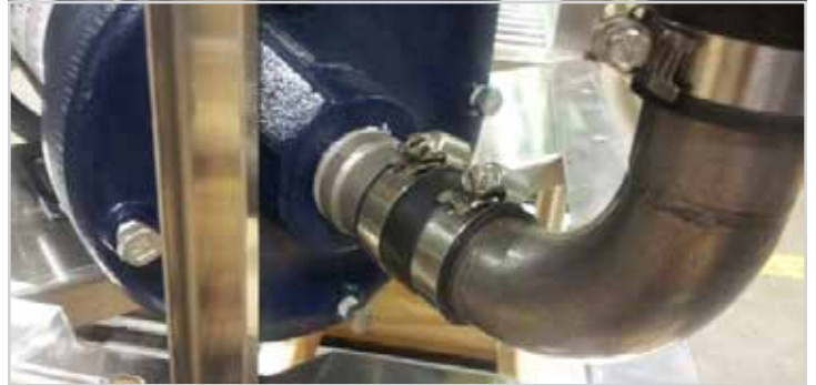
Pump intake and connector sleeves with clamps
