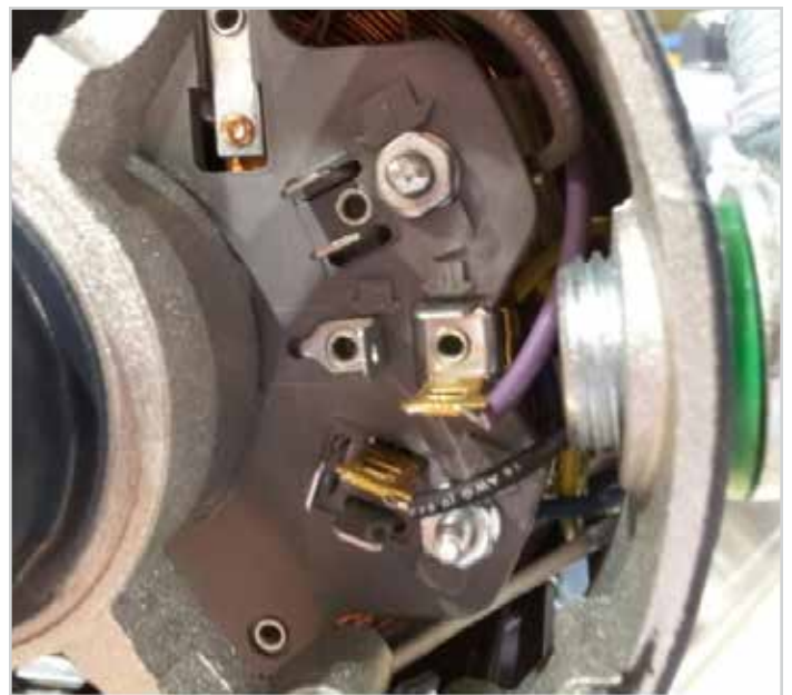
Line connection spades for L1, Neu (arrow 1 & 2)
