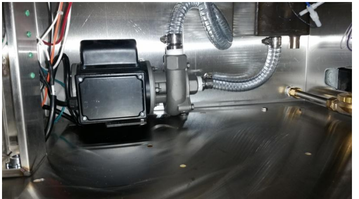
Wash pump with rinse pump removed
