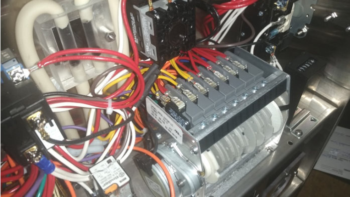
Relays, counter, switches, cam timer, motor contactor
