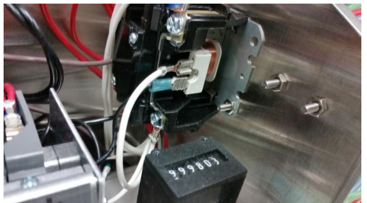
Wash motor contactor next to rack counter
