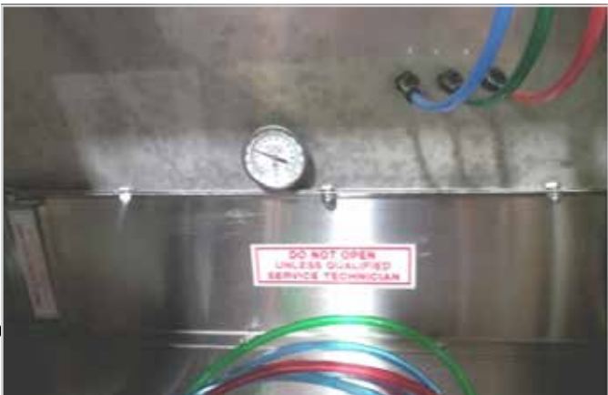
Showing chemical lines and temp gauge in cabinet
