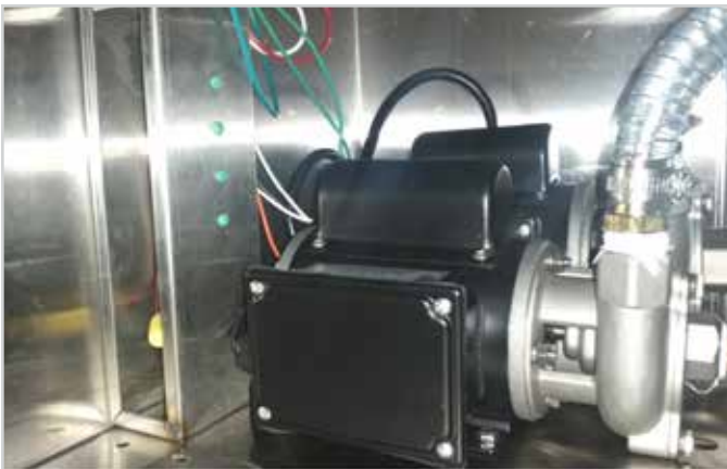
Wash pump is placed behind the rinse pump shown here
