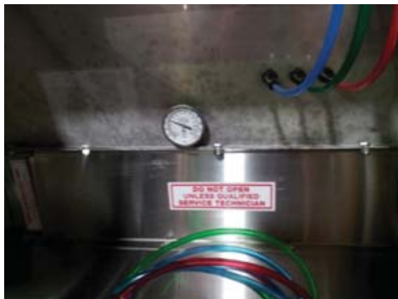
Showing chemical lines and temp gauge in cabinet
