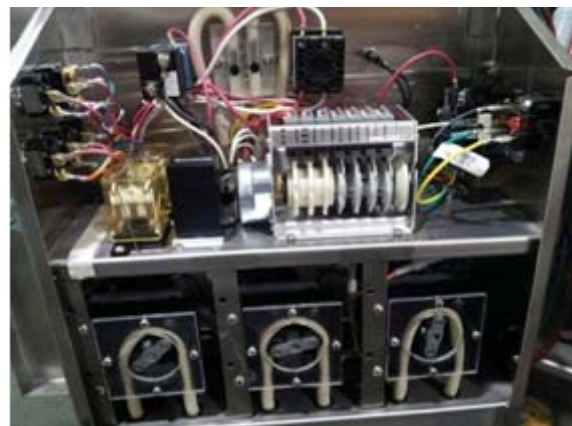
ASQ control box with cover removed
