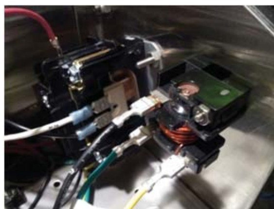
Wash motor contactor and motor relay
