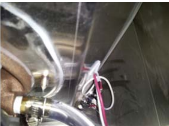
Heater terminals on right rear side of the tank
