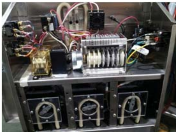
Showing deter, rinse, sanitizer internal chemical pumps
