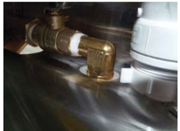
Hot water inlet at ½” elbow
