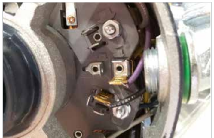
Line connection spades for L1, Neu (arrow 1 & 2)
