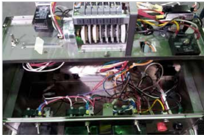
Showing AWS control tray lifted to service pumps
