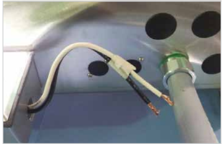
Showing power connection box for 120v wiring
