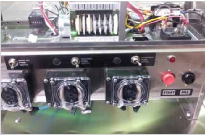
Showing control box, chemical pumps, prime switches
