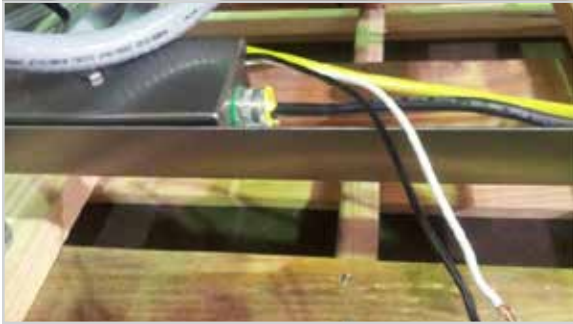
Power junction box for incoming 120v power
