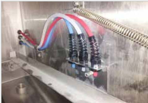
Showing chemical lines above sump
