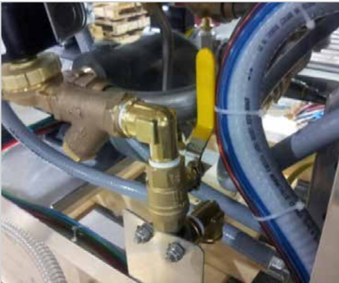
Showing 1/2" female pipe inlet, ball valve, y-line filter, H2O solenoid
