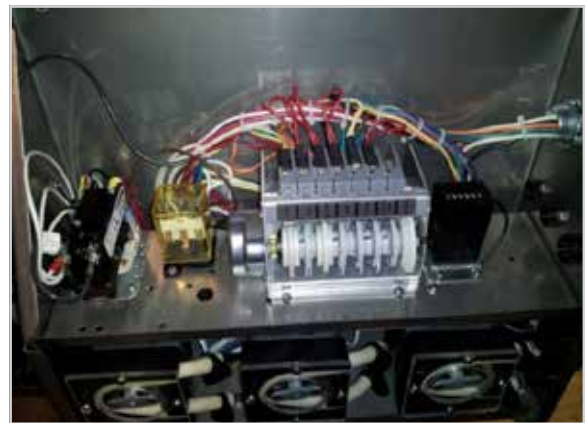
Control box with cover removed
