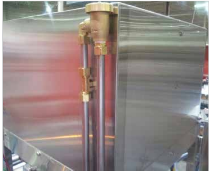
ASSE approved vacuum breaker (backflow preventer)
