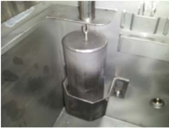
Wash tank float and tank overflow
