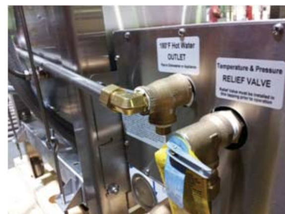
Booster hot outlet line going up to HT-25/34 inlet manifold
