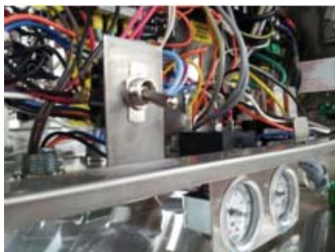
De-lime switch in HT25 control box
