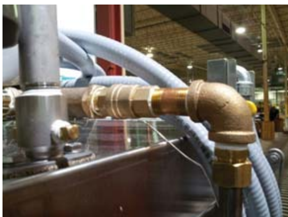
HT hot water inlet ball valve, connected to booster line
