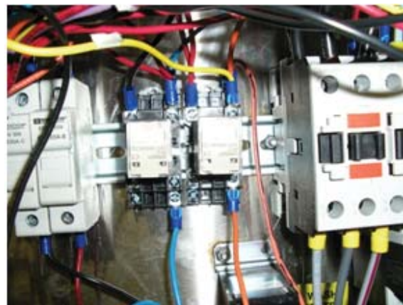
Yellow signal wire from the booster controls heater relay
