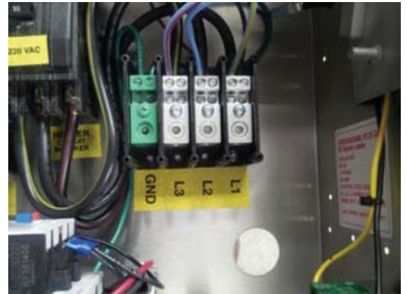
Main distribution block for incoming wire & 1” conduit hole
