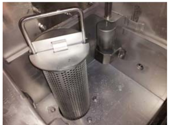
Pump filter in drain sump
