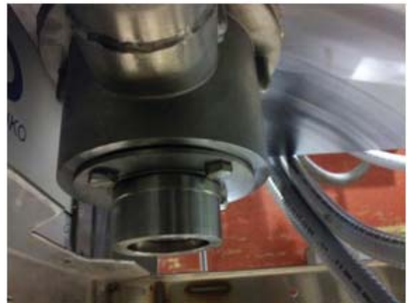
Drain sump connection for copper drain, bottom of tank
