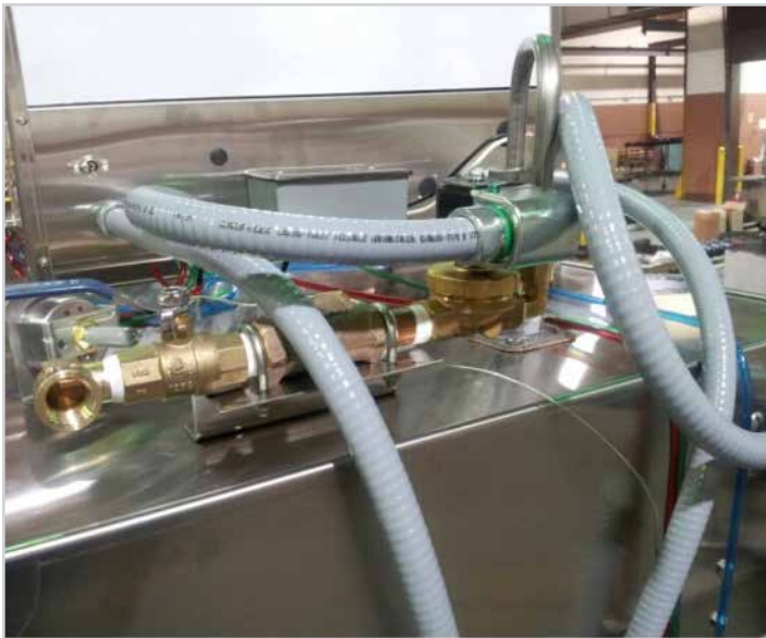
Showing 1/2" female pipe inlet, ball valve, y-line filter, water solenoid
