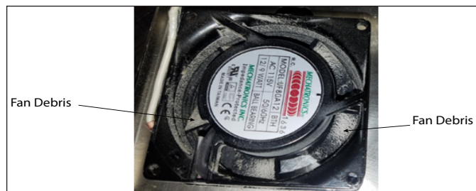
Figure 13. Example of Fan Debris
