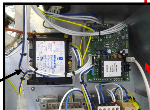
3. Combustion Control board and Blower Control board
