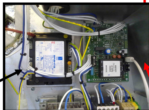
3. Combustion Control board and Blower Control board
