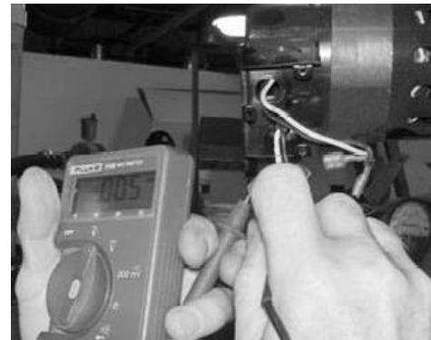
Checking line voltage at the blower wire harness connection on blower.
