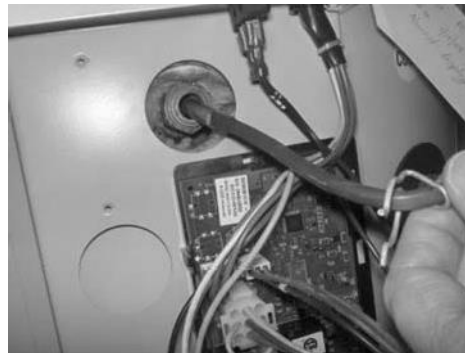
Removing lower sensor from well. Held in place by a clip fastened to well shoulder.
