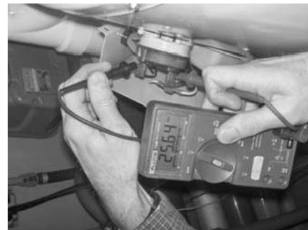
Checking pressure switch contacts. Contacts are open if blower is operating and there is 22-26 volts measured between the two contacts (as in photos)
