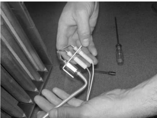
Step 17: Pilot removal for servicing.
