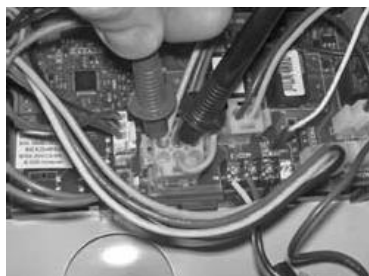
Checking MV pin terminal to gas valve wire harness for 24 volts output to gas valve during heating cycle (pilot must be lit with no sparking).
