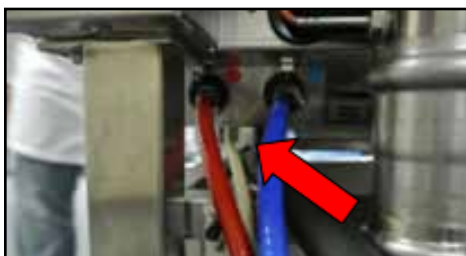
Delime hose runs next to the chemical hose lines.
