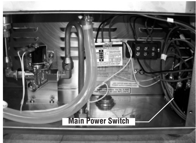
FIG 7 MAIN POWER SWITCH
