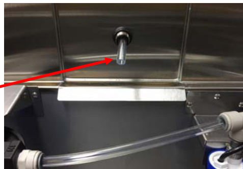
Fig. 5 Zone irrigation nozzle
