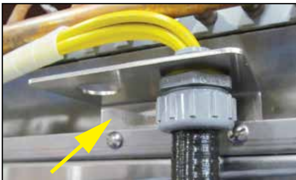
Fig. 3 - Compressor Cable Bracket
