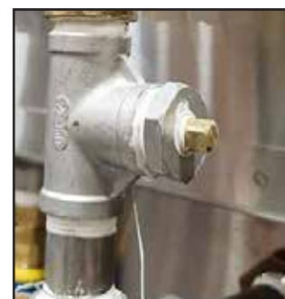
Fig. 22 - Final rinse manifold
