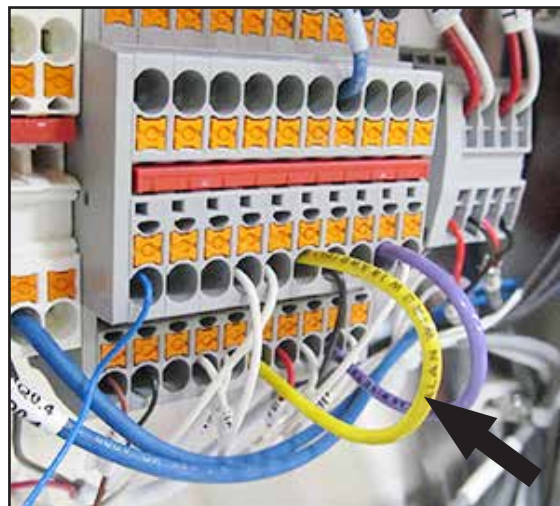
Fig. 7 - Table limit switch yellow jumper
