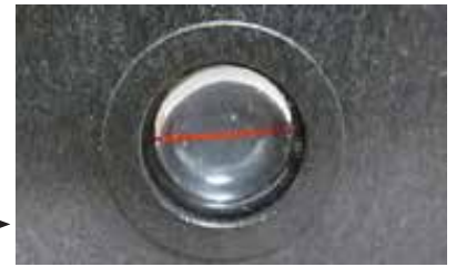
Fig. 77 - Electric valve is closed when red line is horizontal in the valve site window
