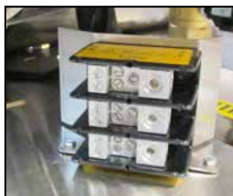
Fig. 3 - Booster terminal block
