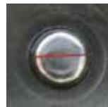
Valve Position Sight Window
