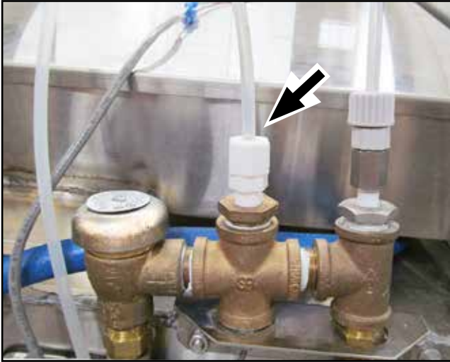
Fig. 20 - Rinse aid injection point
