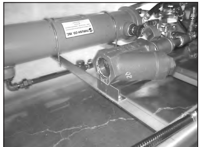
Steam and condensate connection
