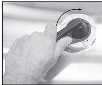
Main Circuit Breaker Switch in the ON position
