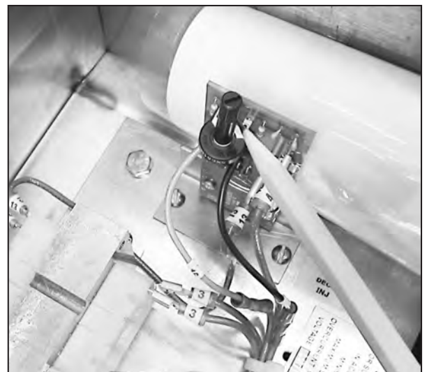
The Deodorizer Injector Speed Control Circuit board is located in the top left corner of the remote control cabinet.
