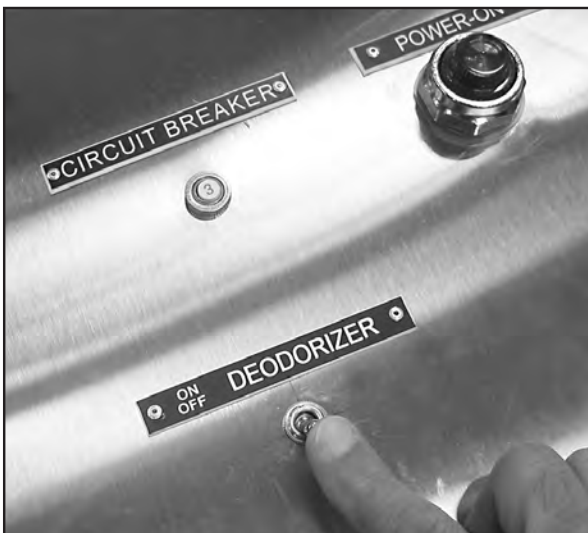
The Deodorizer Power Switch is located on the front of the remote control cabinet.
