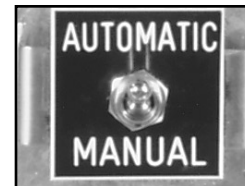
Figure 17 By Pass Switch
