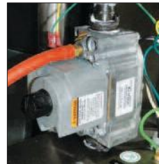
7. Gas Valve (showing hose for Pressure tap)
