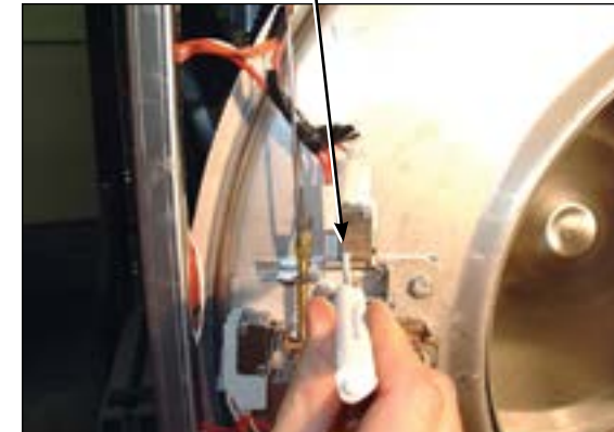
Flat blade screw on door switch latching
