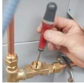
Fig. 7.5 Check if the piston is damaged or dirty, clean or substitute it. Reassemble the solenoid and open the water valve.
