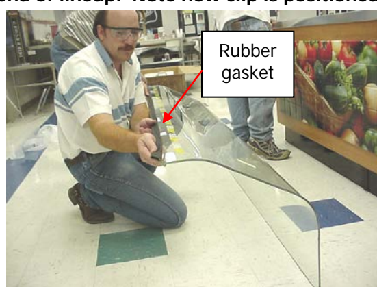
Step 6. Place short rubber gasket onto bottom edge of curved glass. Note orientation of glass in photo. Leave space for U-Channel to fit in center of glass. Put liquid soap onto outside of rubber gasket.
