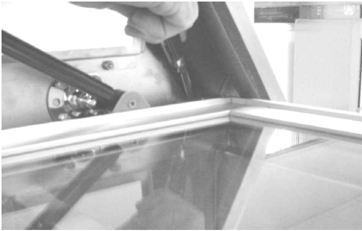
Using a knife or box cutter, score along the edges of the hinge block to loosen silicone sealant.
