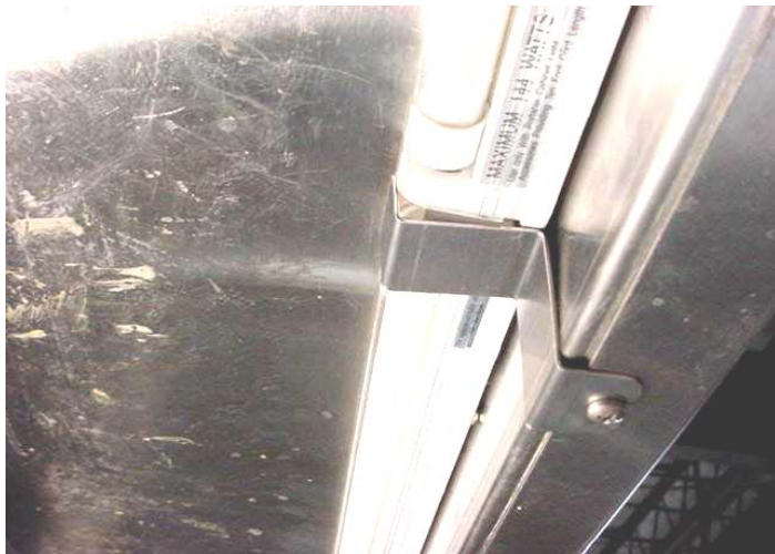
This is a close-up of the installed mounting clip.
