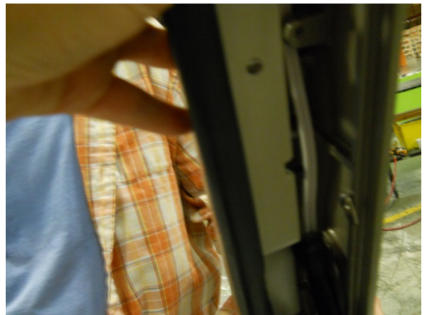
28) Reattach pylon filler being cautious of the light cord in keeping it free from being pinched or in way of screws
