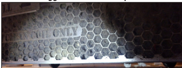
Clogged Filter Needs Replaced
