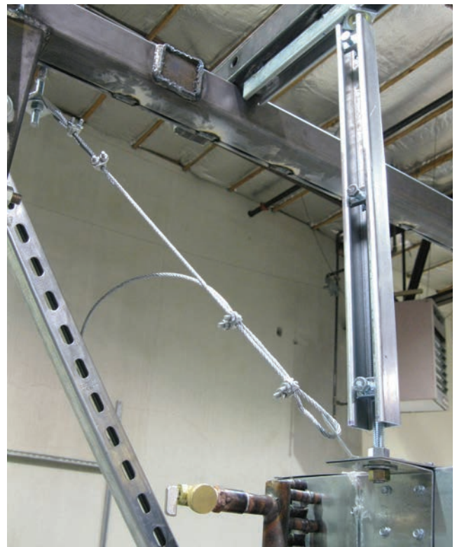
FIGURE 6 – UNISTRUT USED TO STRENGTHEN THE ROD
