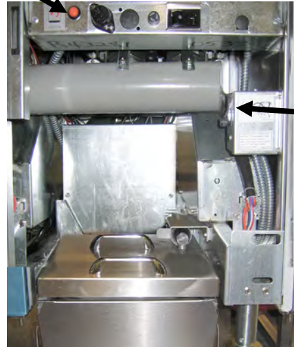
Melting unit power switch
