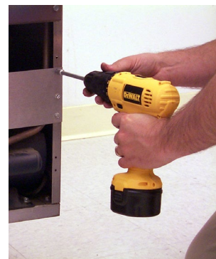
Removing gas manifold shield.
