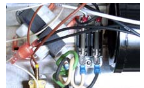
Transformer and fuses.
