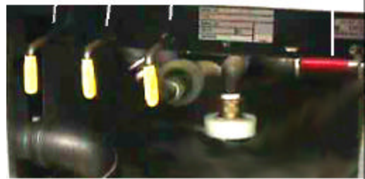
Push-pull variation valve control handles. Yellow handles operate oil return valves, and the red handle operates the hose connect valve.
