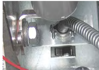
Figure 7 (Rear view of Control Box)
