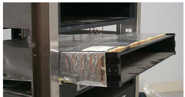
2-7 Figure 11: A faulty slot is slipped from the cabinet.
