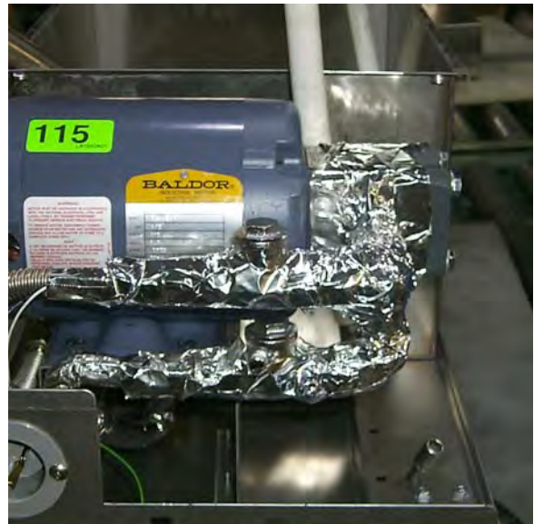
Heater strip installed [115V PF50 (Return/Suction)].
