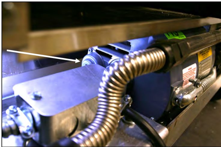
Filter Pump Reset Switch (Arrow)
