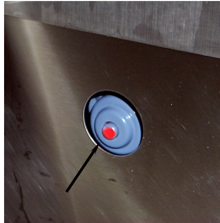
The motor thermal overload switch (arrow) is located on the left side of the filter.
