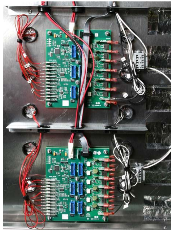
Fig. 7: Distribution board shown with display cables removed.
