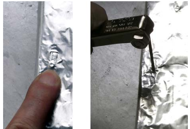
Fig. 11, 12: Find the set screws under the foil insulation and push through with an allen wrench.
