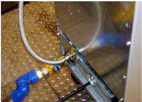
Gas. Water Connections
