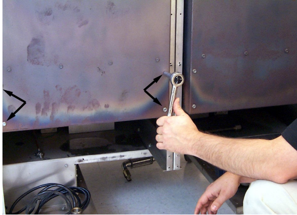
Removing bolts (arrows) securing flue to cookpot.
