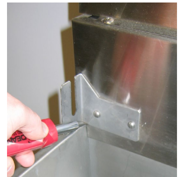
Removing flue cap.
