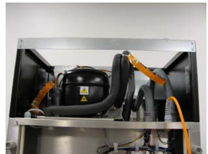
[Photo 2] From rear of unit
