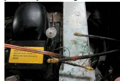
Pinch & solder high side lines or use access fittings on both high & low (evaporator) side.
