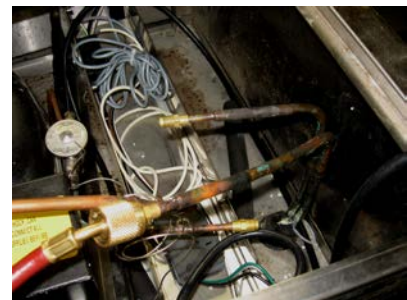
Pressurize the low side to 250 PSIG [17.2 Bars] using nitrogen, check for leaks and pressure level after 10 minutes & again after 24 hours.
