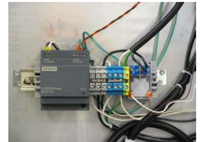
The 24-Volt Power Supply is DIN rail mounted on back of unit.
