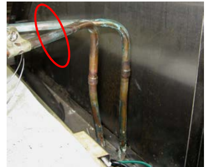
Separate and cut the high & low side lines from the (cold wall) evaporator and solder on access fittings.
